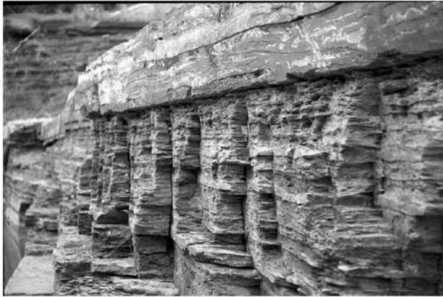
Figure 1. A set of parallel joints in the alternating siltstone and shale beds on the Appalachian Plateau near Finger Lakes, central New York (courtesy of Bruce Carter; see also Helgeson and Aydin [1991] and Engelder et al. [1999]).
