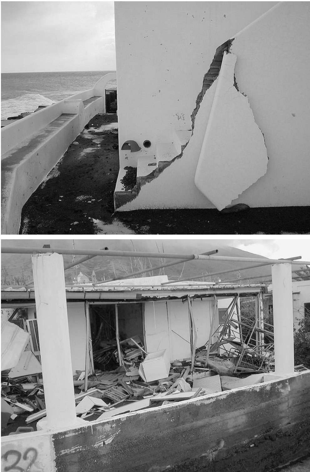
Fig. 11 a Typical damage observed to holiday houses in Punta Lena which were built very close to the shoreline. The picture was taken during the second of the three surveys (21–23 January 2003). b Another typical view of damage produced by the 30 December 2002
