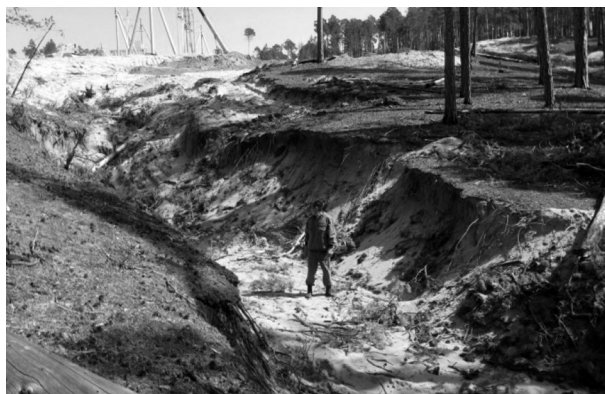
Fig. 2. Thermoerosion along the ESPO pipeline. Photo by I.V. Dorofeev.
