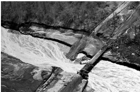
Fig.5. The road and the dam in the area of river Bekesh were destroyed with mud flows. Photo by Yu.V. Demyanchuk.
