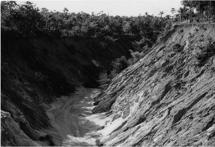
Fig. 10. Large (ca. 15–20 m deep and ca. 30–40 m wide) permanent gully which developed in unconsolidated Tertiary sandy sediments, Owerri, South Nigeria (April 1988). The development of such gullies leads to enhanced subsurface drainage (water table lowering) of these hillslopes.
