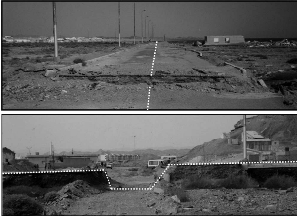
Fig. 9. Part of the pedestrian walkway damaged by a flood in 1996. The line annotated runs along the length of the walkway and shows the general vertical profile after the flood damage in the bottom image.
