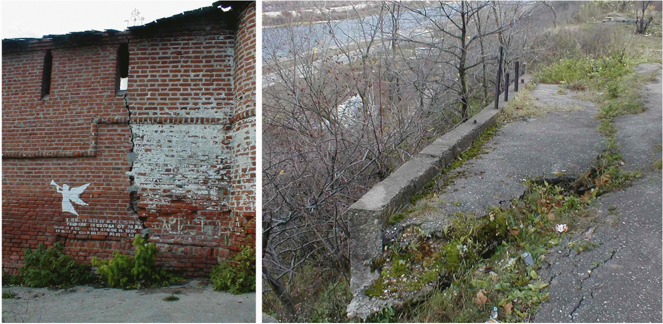
Figure 5. A crack near the foothill of the Pechera monastery that broke the wall.
