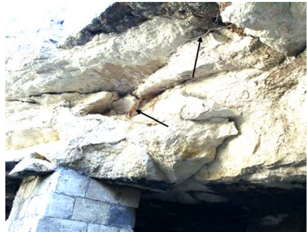
Fig. 8 Roots on the roof of the collapsed cave in Hamdi Kutlar Street
