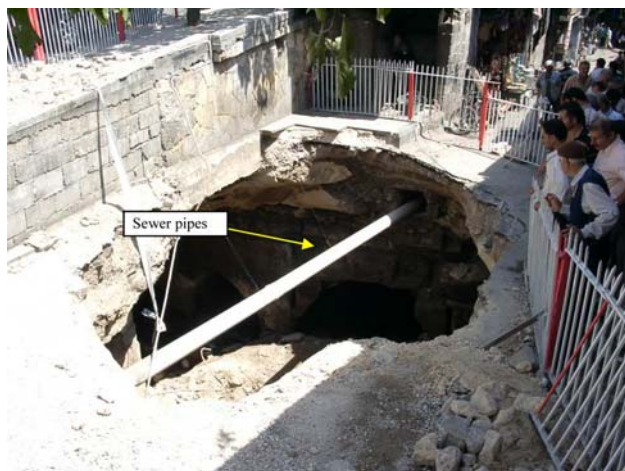
Fig. 3 General view of the collapsed cave in Hamdi Kutlar Street
