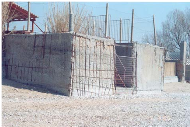
Photo 10 Nea Chili. Failure of hard protection measures
