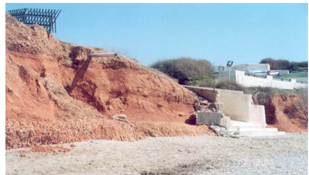
Photo 8 Coast erosion at Hilli Village. The destruction of the fence and the stairs and various layers of conglomerates are distinguished
