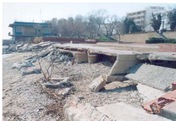
Photo 12 Destruction of an open recreation plateau, outside of the Sea-Scout Center at the west side of the Alexandroupolis City Port, in 2004
