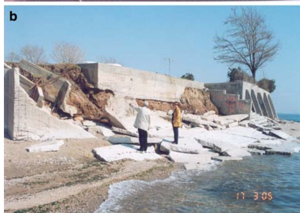
Photo 11 a Aerial photo of Alexandroupolis City coast at recreation club “ARGO”, after the construction of a retaining wall, in 1990s for the coast protection. b Destruction of part of the retaining wall of the coast, at recreation club “ARGO”, from sea (storm) waves in 2004
