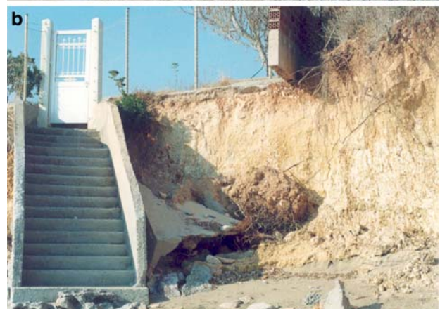
Photo 5 a, b Coast erosion west of Hili Village affecting human structures
