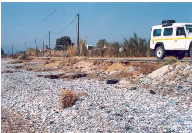
Photo 2 Erosion of the road pavement at Dikella
