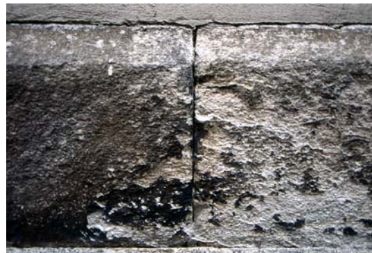
Fig. 3 S. Jorge church, La Coruña. Sampling area: close-up of thin black sulphated layer on granitic surface. Note also the presence of white powdery efflorescences on the same surface
