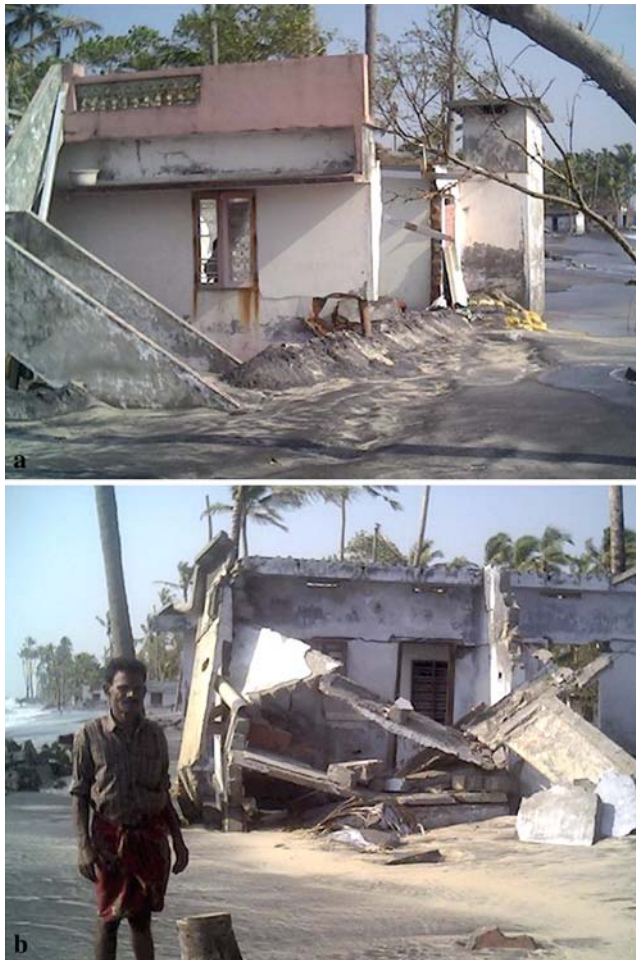
Fig. 2 a, b Damaged house and huge deposition of black sands in the settlement area near Valiazhikal due to tsunami waves
