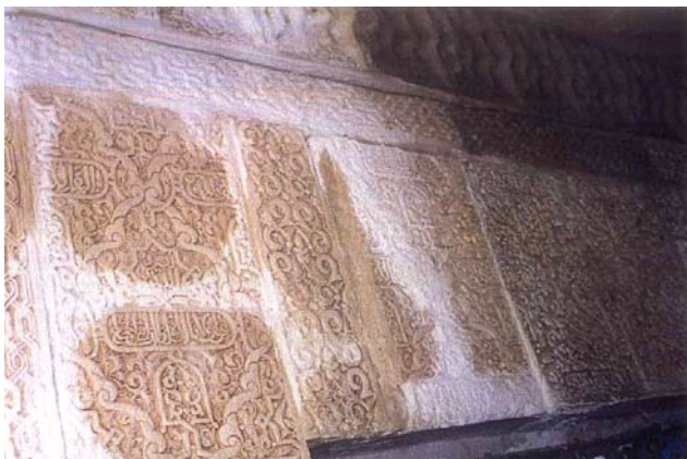
Fig. 4 White salt efflorescence on the Islamic ingaves at Al-Cazaba Palace, Al-hambra
