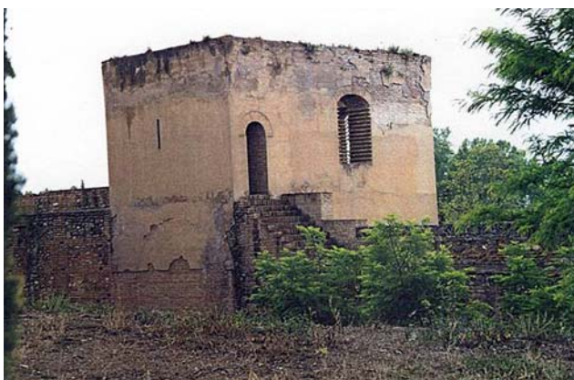
Fig. 6 Narrow single to map cracks at some parts of Al-hambra, 35% of the surface render are obliterated, tiny plants grow up through these cracks
