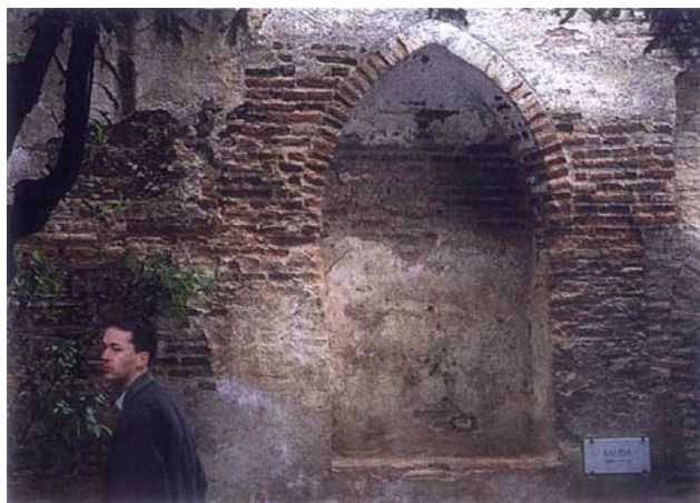
Fig. 3 Stone surface disintegration, damp stone surface and obliteration of surface render at Salida, Al-hambra structure
