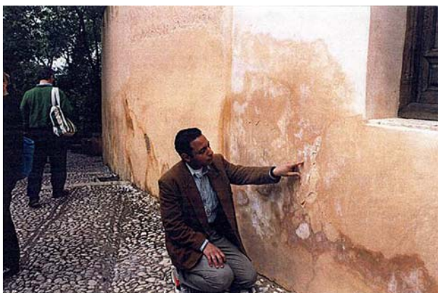
Fig. 5 Damp stone surface, pop-outs, white salt efflorescence and render obliteration noted on wall side of Al-hambra
