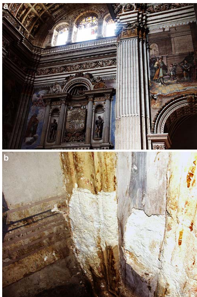
Fig. 1 a Monasterio de San Jerónimo, Granada. Interior view of Church (Capilla del lateral Izquierdo del Crucero). b Monasterio de San Jerónimo, Granada. Detail showing salt damage to stonework and wall paintings within church interior
