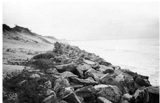
Fig. 7 Riprap to protect cliff. But the erosion process has continued in the upper portion
