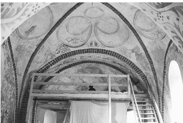
Fig. 2 View of the inside of the chancel looking towards the apse. The vault is a 250 mm thick masonry structure, contemporary with the outer walls
