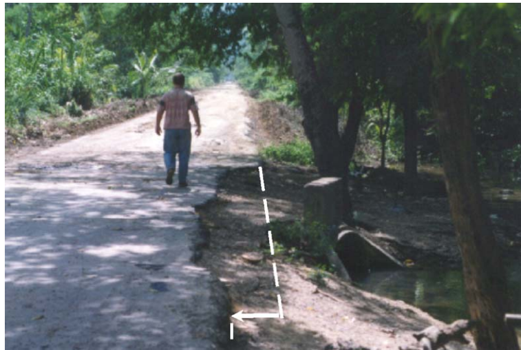
Fig. 9. Maximum coseismic slip of 40 cm observed on a rural road, adjacent to a concrete drain that deflects and concentrates all slip along a single plane. This locality is west of Pantoño and about 1 km north of national road 10 (refer to Fig. 1 for location).
